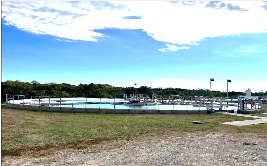
Upgraded Middle Final Clarifier
