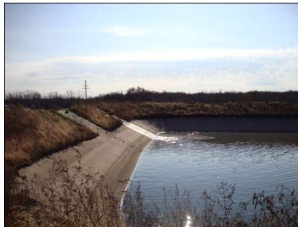
Pumping to FEQ—looking south
