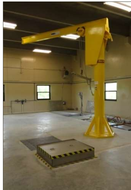
Jib crane (pits for acid wash)
