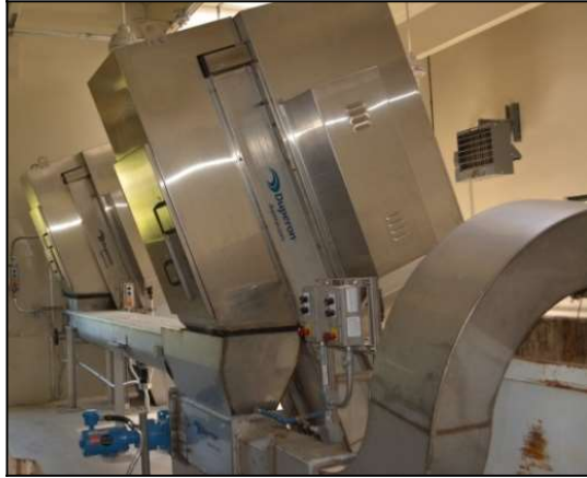
Screens—upper level with compactor
