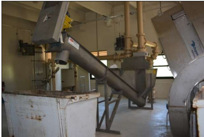
Grit auger, main floor
