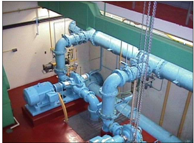
Inside of the Miami Street Pumping Station
