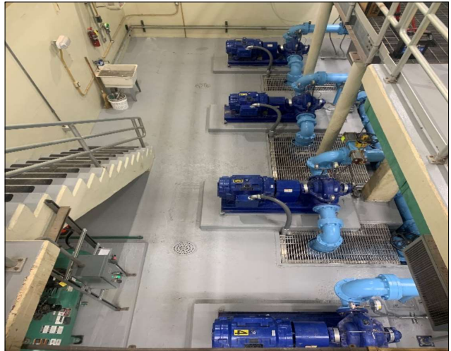
Inside the North Street Pumping Station
