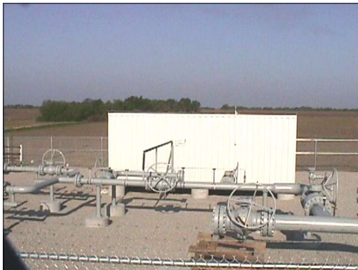
Panhandle meter site, odorizer building
