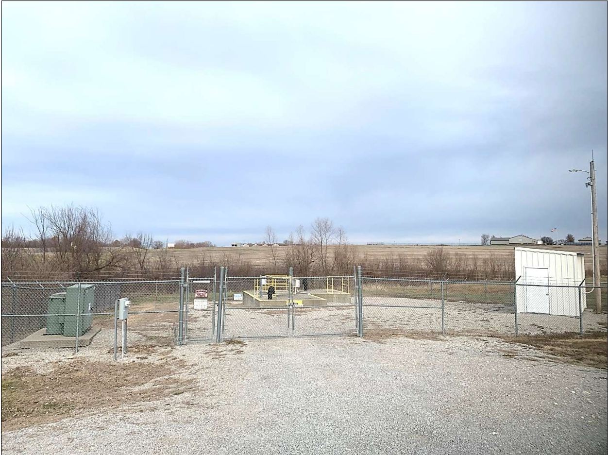
South Odell Lift Station
