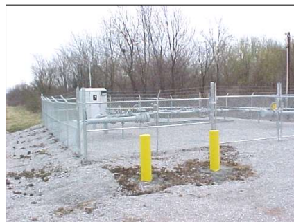
MME meter station, looking east
