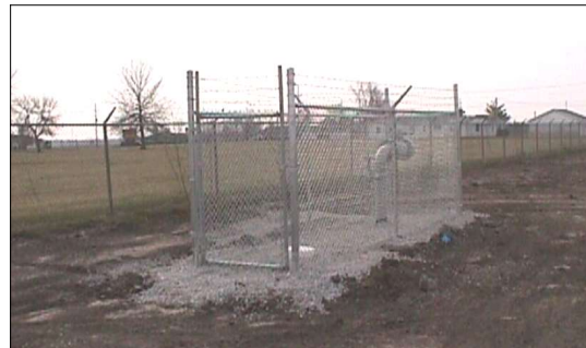
Control Valve with Tee and Valve for Future Development
